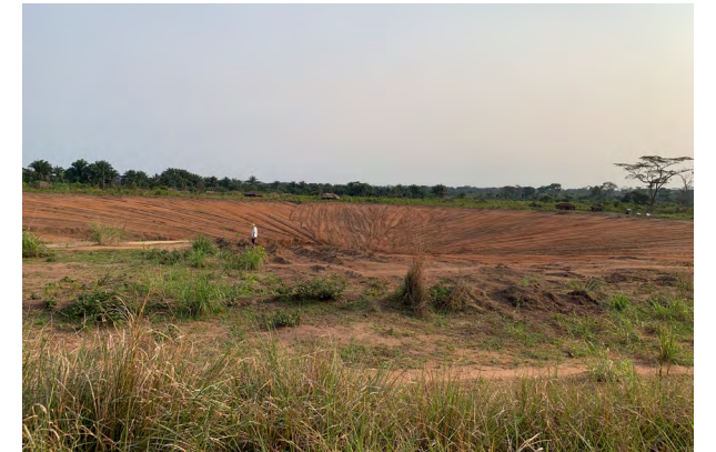
Borrow pits refilled and graded to a gentle slope at the 87-km Road Project in the Democratic Republic of Congo
