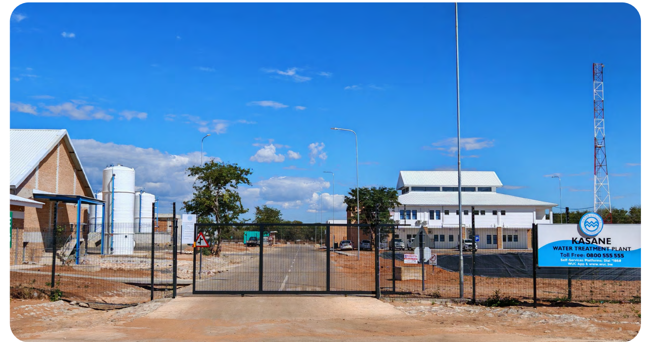
The team at the Kasane Water Treatment Plant Project in Botswana adhered to lean management principles, carefully planned the construction sequence, and successfully completed all tasks, earning unanimous recognition from the client and supervisor
