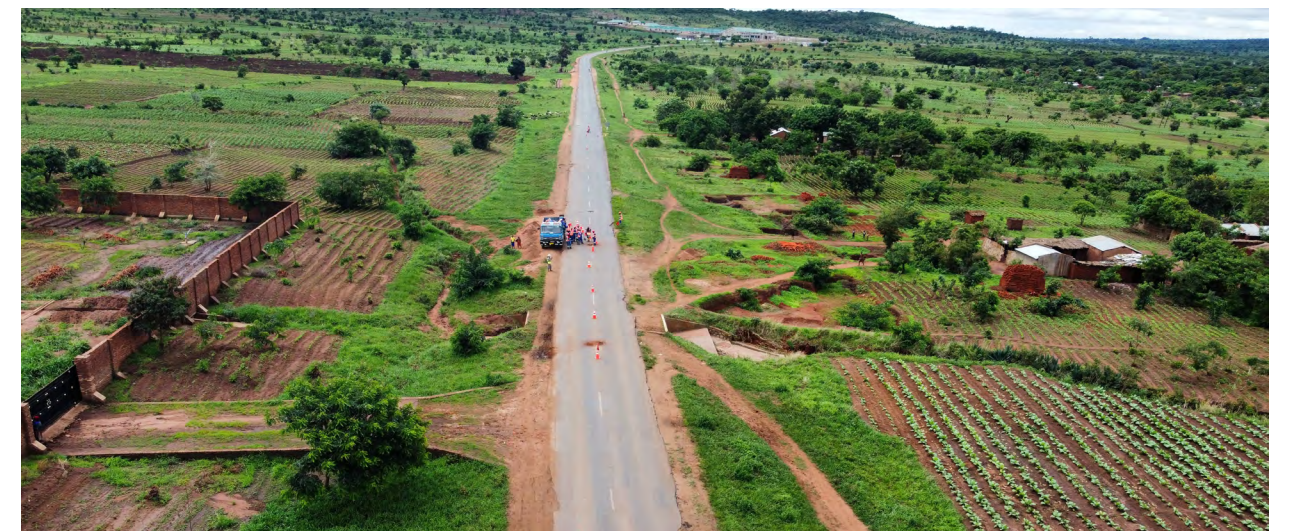
CJIC developed and implemented an environmental protection plan for the Malawi M1 Highway Project, which included measures to protect local wildlife and vegetation along the route.
